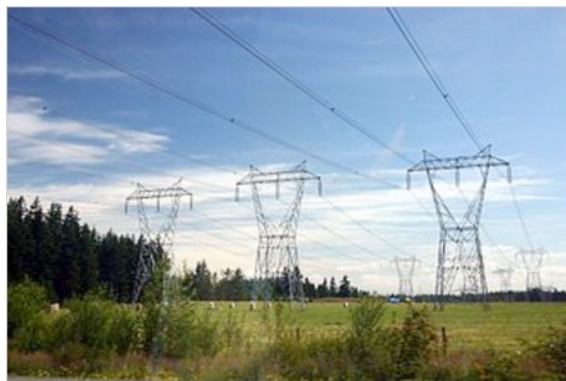
Three-phase electric power transmission lines
